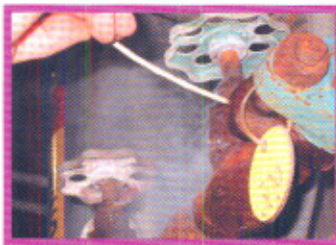
A sulfur stick also is useful for finding smaller leaks.
