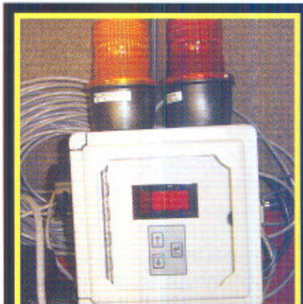
Alarm systems can produce both visual and audible warning signals to alert those in the area that dangerous levels of ammonia concentration have been reached.
