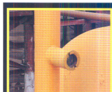
Sight glasses are common sources of ammonia leaks.
